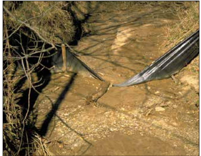
Silt Fence Failure: Accumulated sediment released in a mass failure
